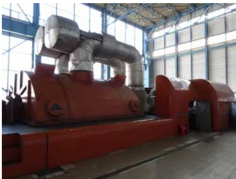
Power house and turbine
